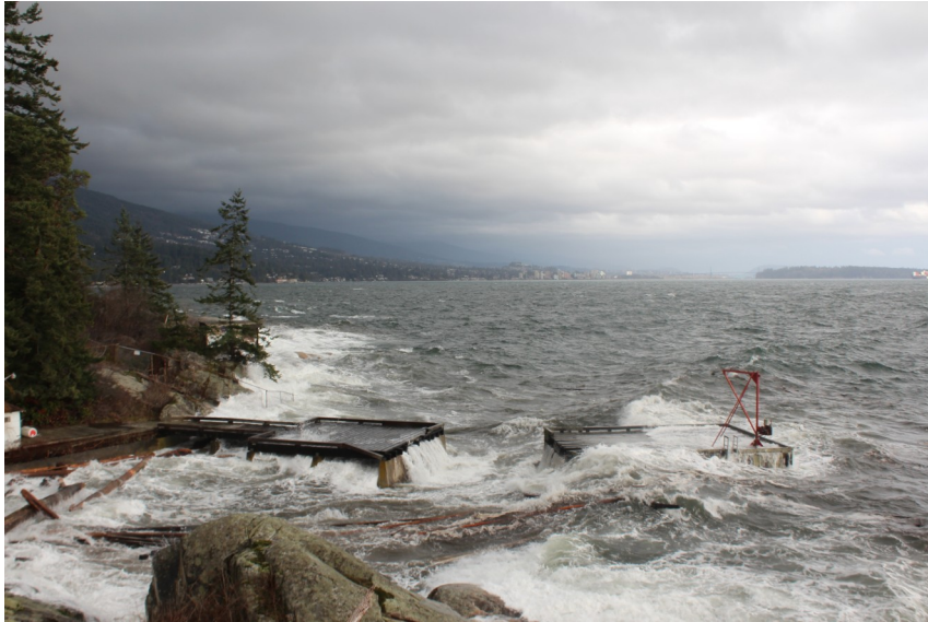
High waves during December 20th's storm destroying the mid-section of Point Atkinson's dock. Fisheries & Oceans Canada engineers inspecting the dock after the storm said the dock will be rebuilt. Photo: Elaine Graham
